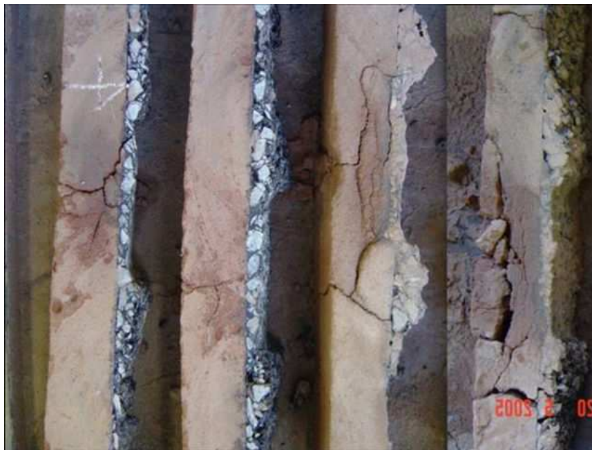
40 FIGURE 3a Side view of beams taken from 3 percent cement section. Note different phases of failure.
