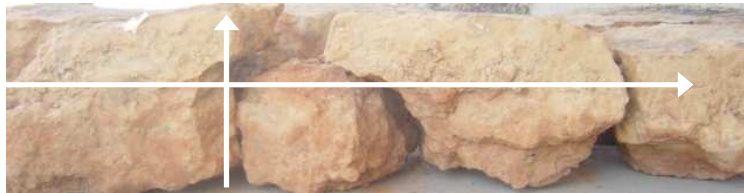
FIGURE 10b Elevation View of the CTB slab extracted from full-scale test section 4 for diagnostic investigation (160x1200)
